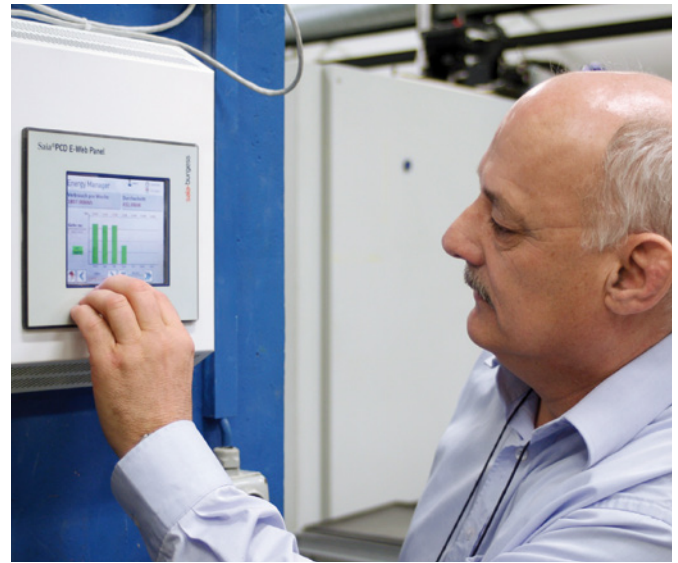
Erwin Brügger monitors various processing data with the help of a Saia PCD e-Web panel in the production hall, including the energy consumption of every individual injection moulding machine.
