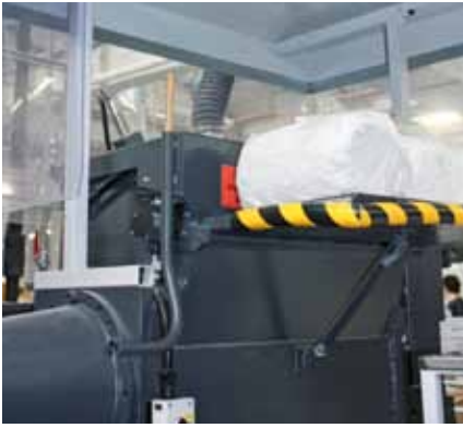
The loading capacity of the poly-stuffer is three BMC bales which are loaded manually.
